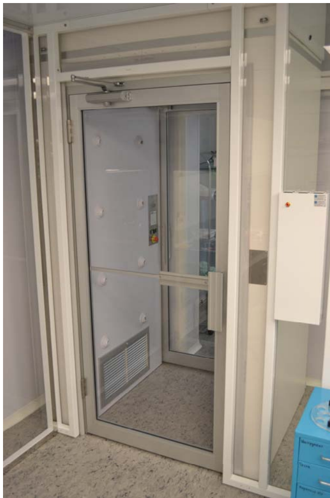
Clean Room – View 3
